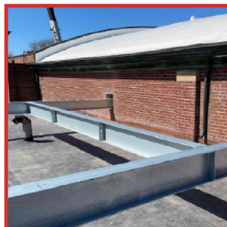
Steel supports for one of the rooftop HVAC units has been installed.
